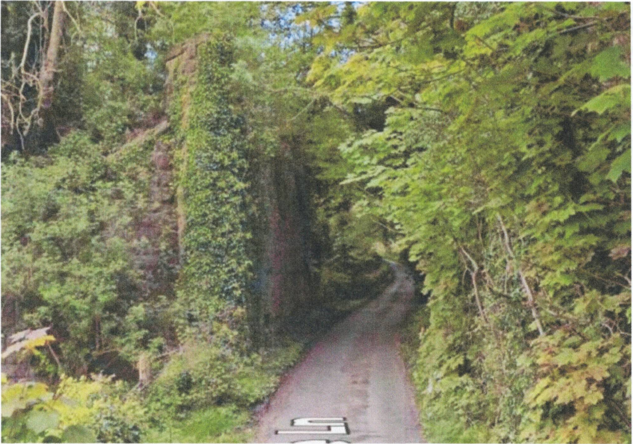
The remains of the railway bridge over Wellhouse Lane seen from the Northeast. The northern abutment is hidden by vegetation. The Montgomery Canal, in its overgrown state, is off the right side of this image. [Google Streetview, April 2024]
