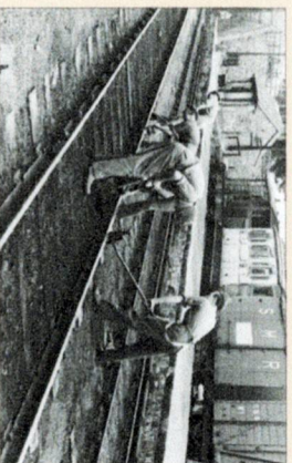
Kimmerley Station. The Permanent Way gang attending to the packing of a length within Kimmerley Station. Two vans of the breakdown train were in the bay platform - the nearest lettered 'S.M.R. No 1 WD Breakdown Train' - together with the ex-L&SWR Royal Saloon No 1A and a WD standard brake van. Image: David Peterson, from the Detachment Photograph Album.
